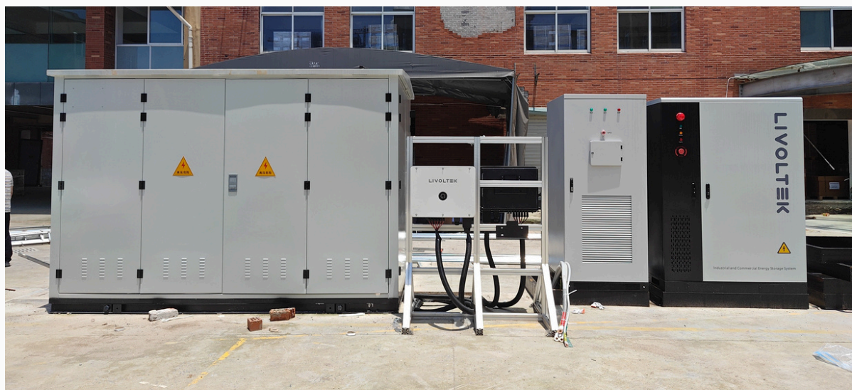
Our Grid Tied Inverter & PCS Unit
