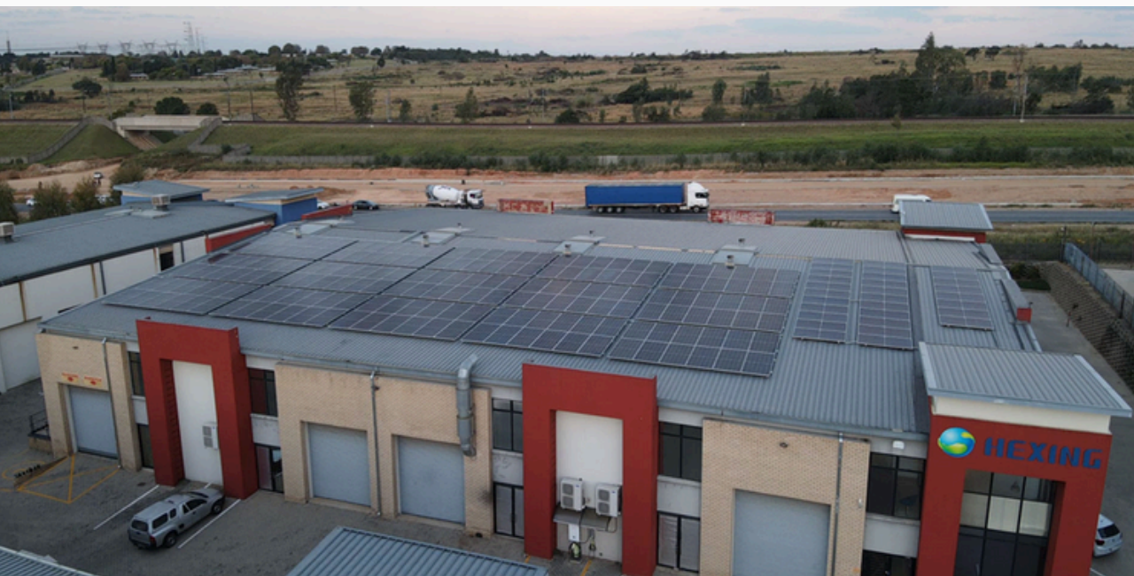
Aerial view of our completed solar power installation at Hexing
